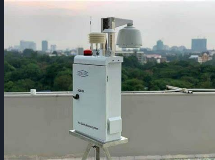
Image of Air Quality System
